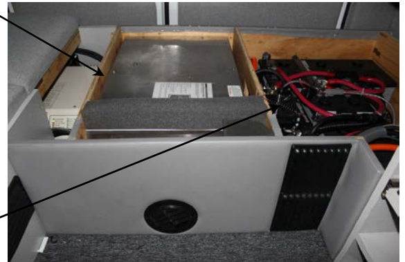
DEDICATED BATTERY BANK
